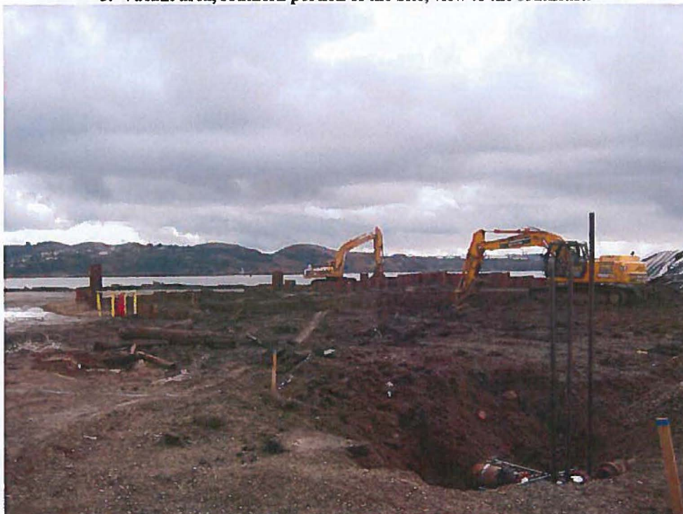
4. Excavation and stockpiles on western portion of the Site, view to the west.
