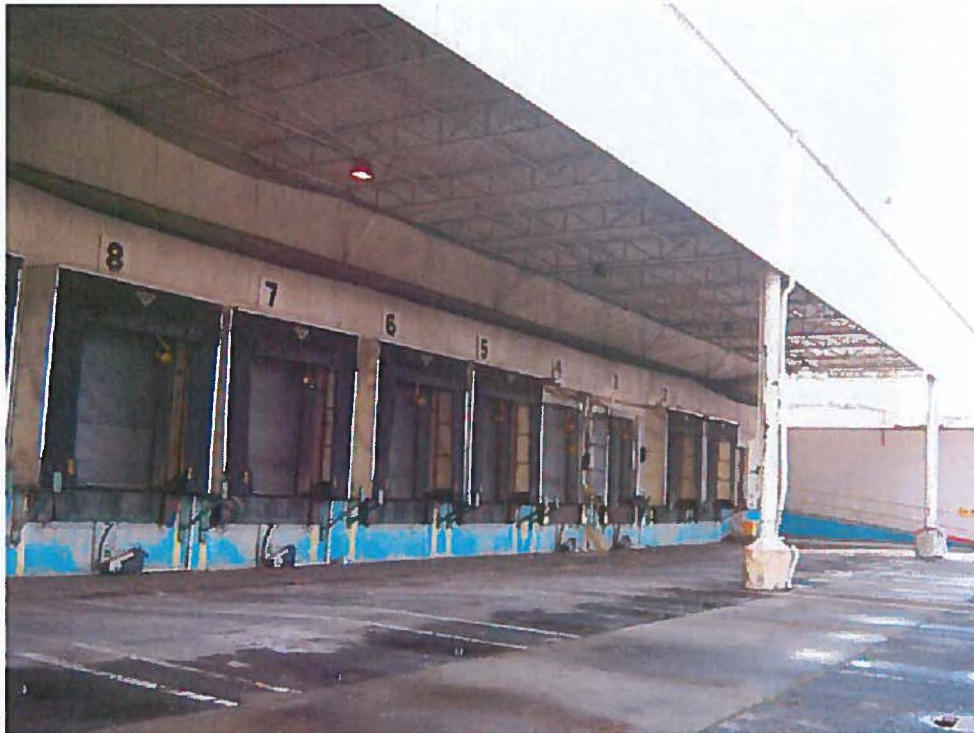
11. Loading dock area on northern end of New Warehouse building, view to the west.
